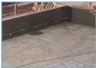
Bund before relining
